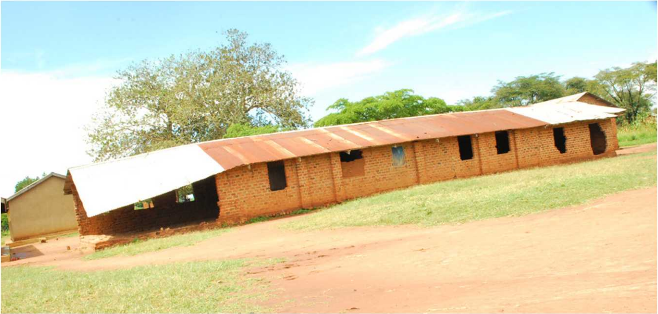
The Community Monitors are now lobbying for the reconstruction of this classroom at Katiry Primary School block which collapsed due to heavy rains
