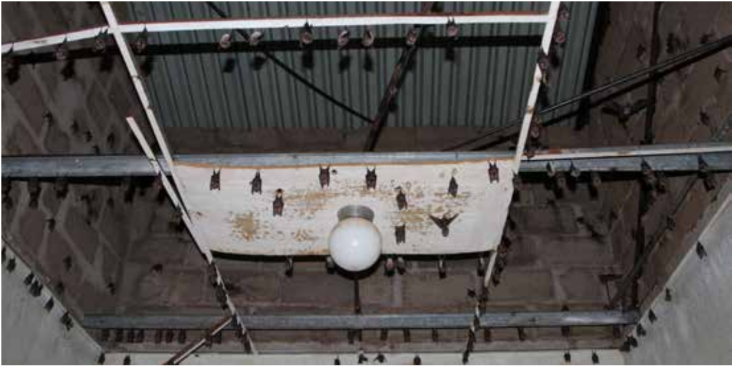
Bats have made Abim hospital their home. A tour of Abim hospital during the Anti- Corruption caravan in Abim district on 7 th - August- 2014, reveal a medical facility that corruption has driven to rot with no medical services; equipment, medicine, water, human resources, electricity and all left to whom it may Concern. Residents wonder why they continue to pay taxes when the Government has abandoned the district with no service delivery.
