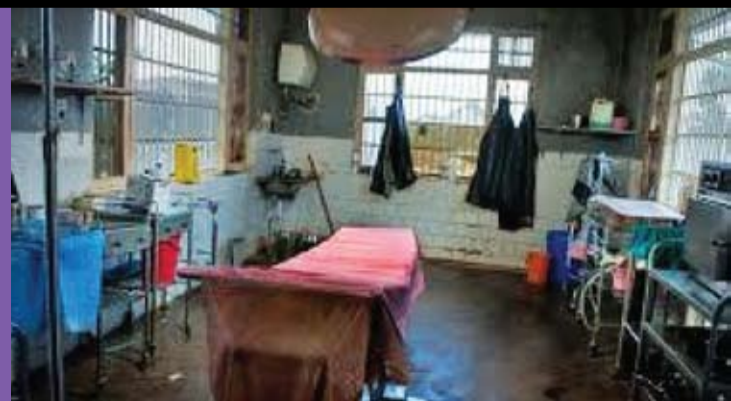
Dilapidated operation theaters in referral hospitals
