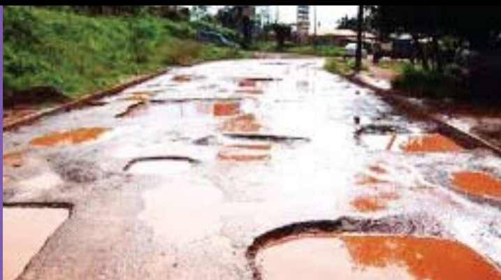
Pothole-filled City roads
