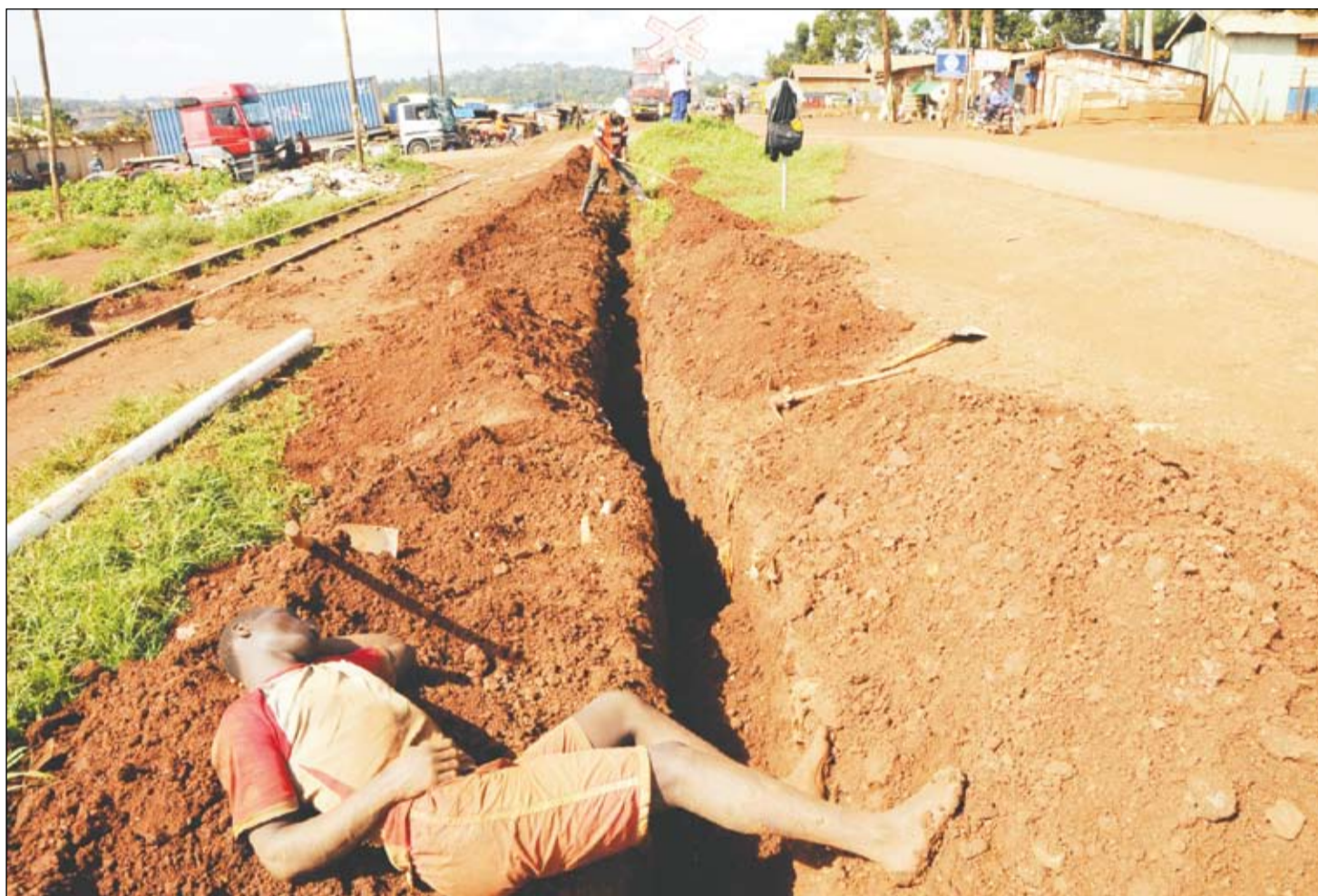
A youthful casual labourer takes a nap during a long day's work digging a trench for cables near Nakawa Magistrates Court in Kampala.
