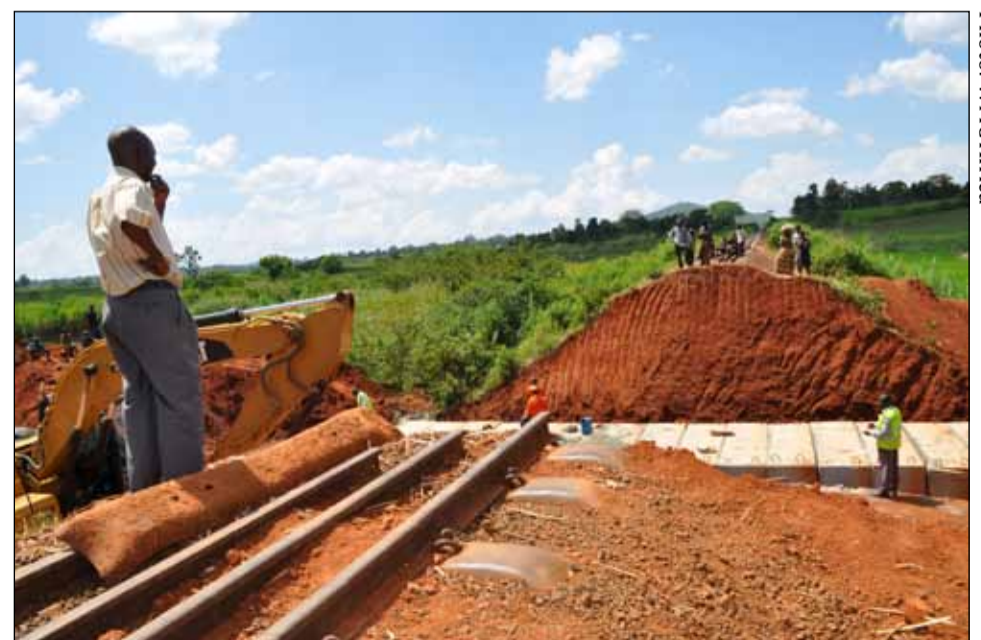
Repairs to the railway network operated by RVR in Kenya and Uganda: a modest start to getting the region ready for oil production.
